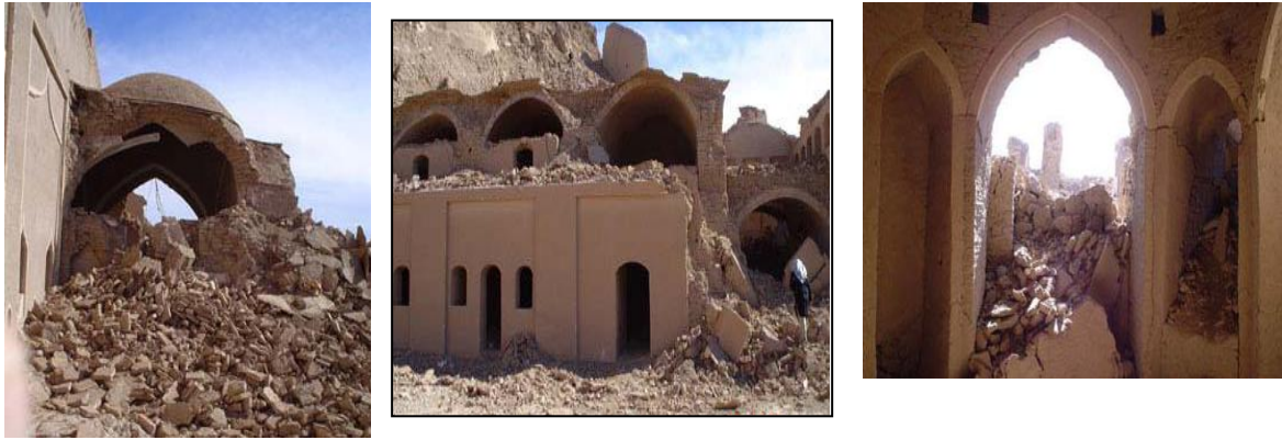
Fig. 3: Performance of arcs, vaults and domes the 2003 bam earthquake (Mahdi, 2004)
